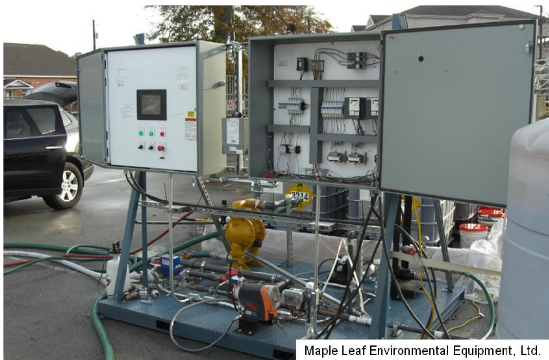
Figure 5-14. Automated process control system.
